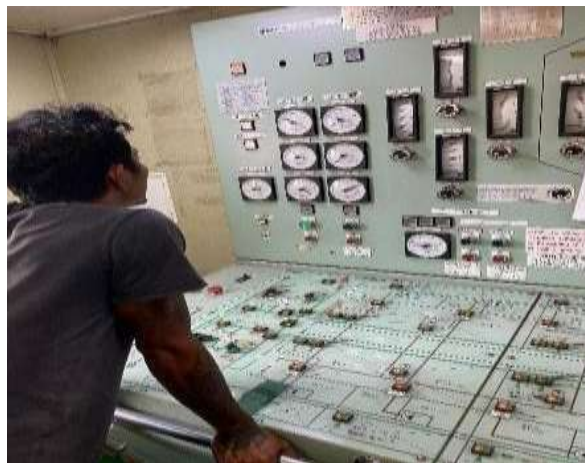
Picture 4. Ballast Control Room
