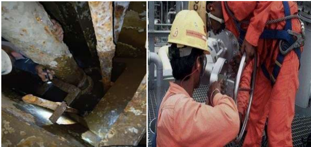
Picture 7. rust found in ballast tank and valve ballast
