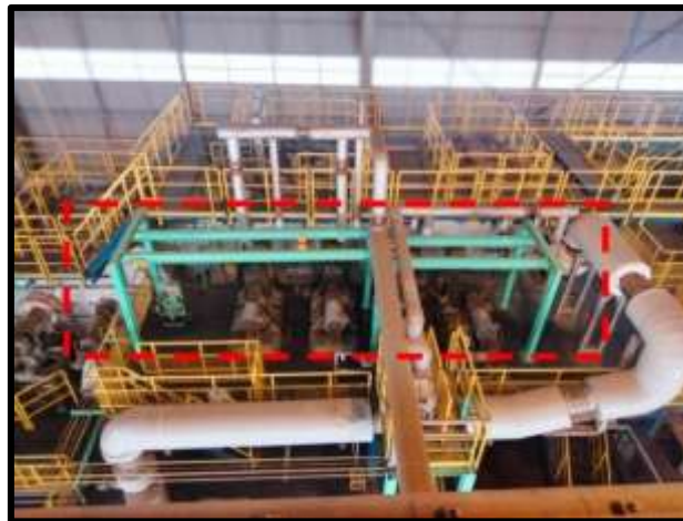
Gambar 3. 5 Implementasi Gantry di Area Furnace Sumber: PT. XYZ, 2025
