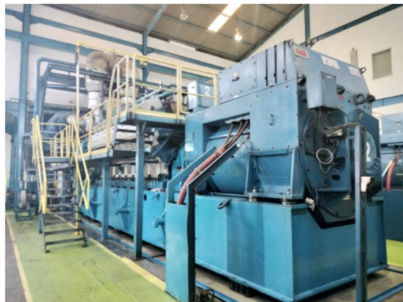
Figure 1. Electric Energy Generation Machine Wartsila Engine Control System
